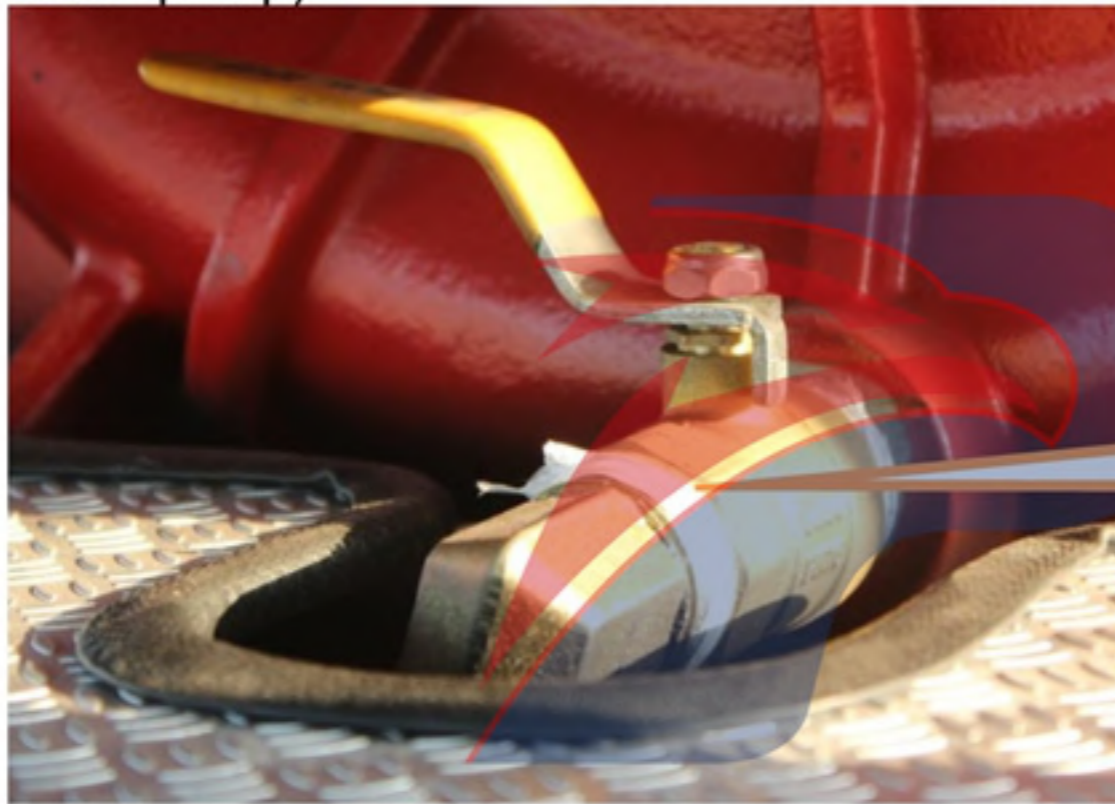
Pump Drain Ball Valve, connected with pipeline
